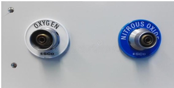
Oxygen & Nitrous Oxide wall outlets
